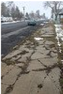
Damaged sidewalks can make walking unpleasant and unsafe.
